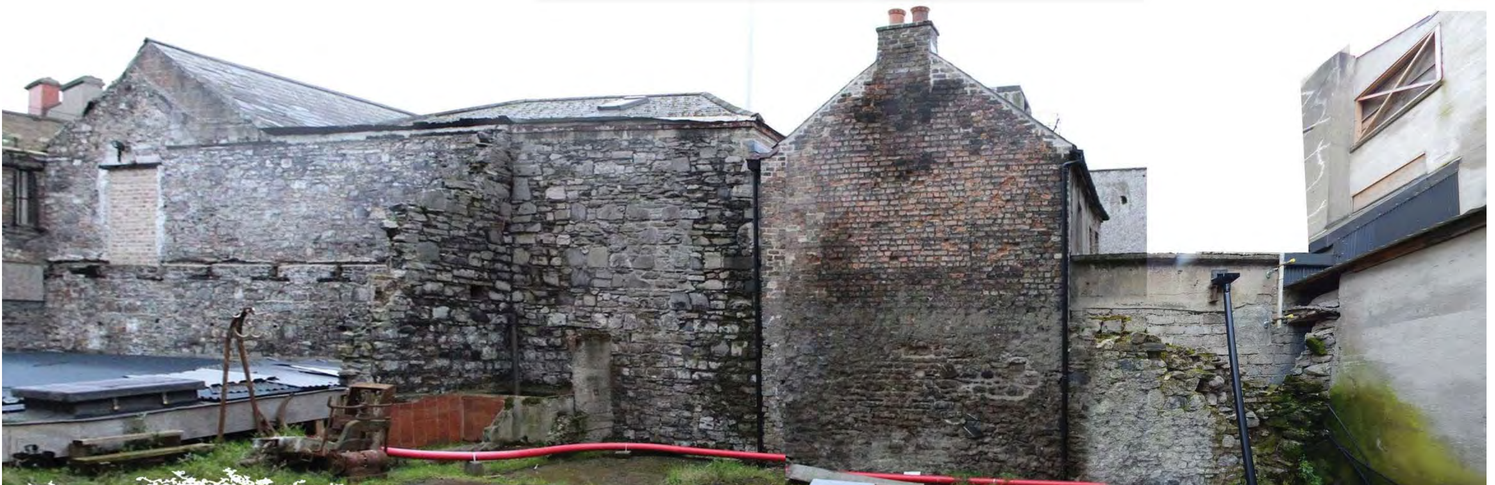
05. Stone wall along No. 14/15 - differing roofscapes along divided leased plots of land
