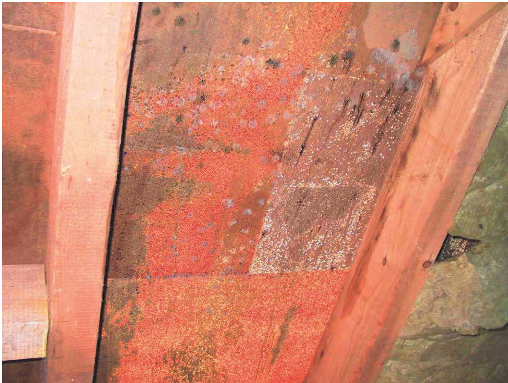
Image 2: moisture accumulation behind sarking board and resultant mould following wet trades
