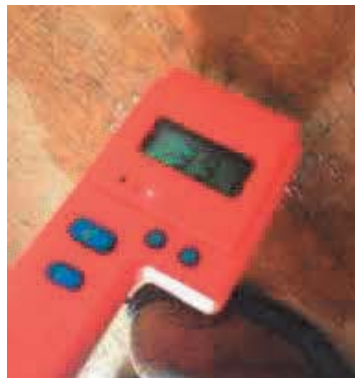
Image 1: A moisture meter reading on site inspection reading a moisture content >30% in OSB3.
