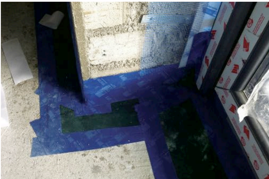
Fig 5.3 Achieving airtightness: (Top) First floor ceiling removed and airtight membrane installed below the existing roof joist, with battens to form service cavity, membrane taped to internal wet plaster layer. (Middle) Ground floor ceilings removed and internal plaster layer patched between floor joists, joists ends taped at wall junction. (Bottom) Airtight sealing tape to junction of all external walls and new concrete floor slab. Passive House certified windows, taped at all junctions to form continuous seal with internal wet plaster layer. (Source: McGuinness, 2014).
