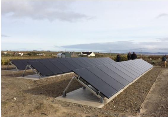
Fig 4.9 Eachléim PV Installation
